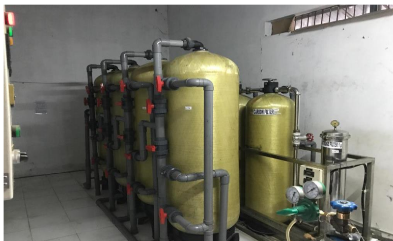
Gambar 1.1 Water Treatment Plant di PT. Bharata Sakti Persada
